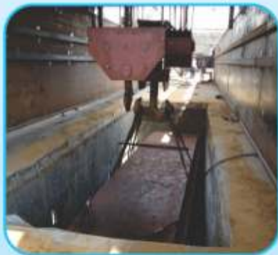
100 T Crane testing at works
