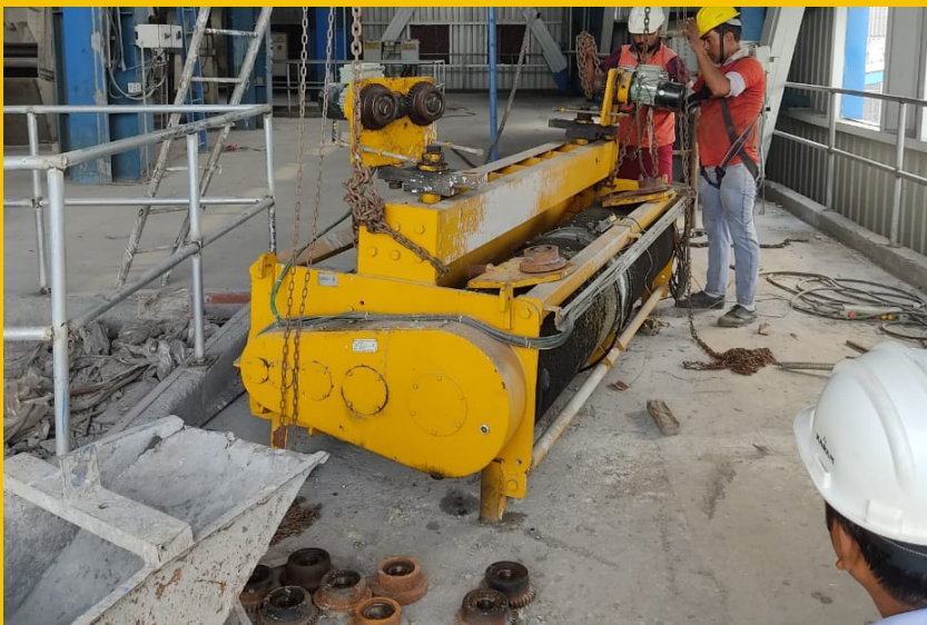
Hoist in preventive maintenance
