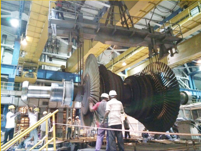
During overhauling Turbine lifted by REVA Crane (105MT) at NTPC Mouda (2*500MW+2*660MW)
